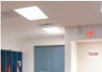
Exit and Emergency
